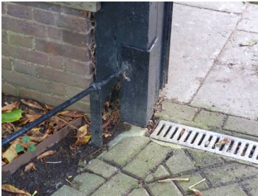
Rotten oak post adjacent to drainage channels (2.20). Steel reinforcement bolted to brickwork(2.21)
