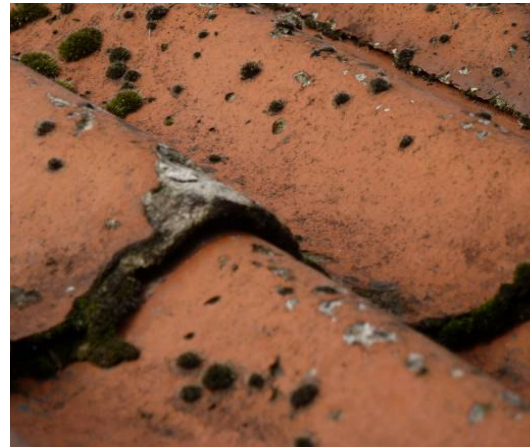
Friable roof surface (4.14)
