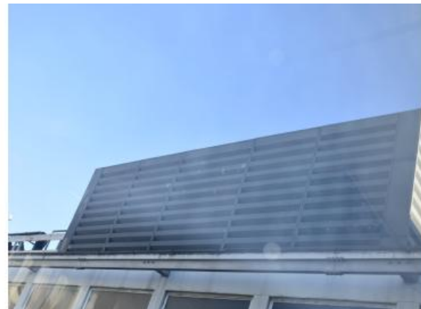
Image 6: Existing Plant SScreen
