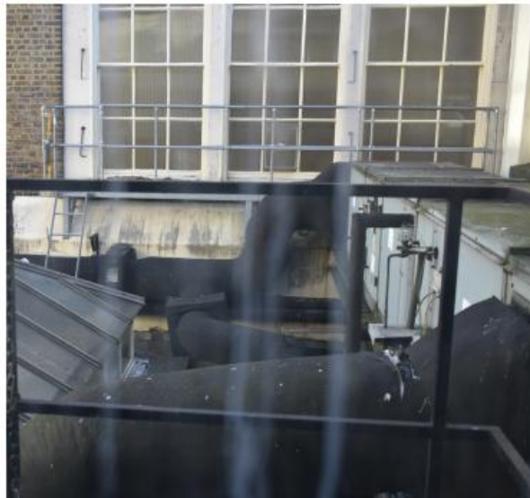
Image 2: Existing Plant Above the Robing Room
