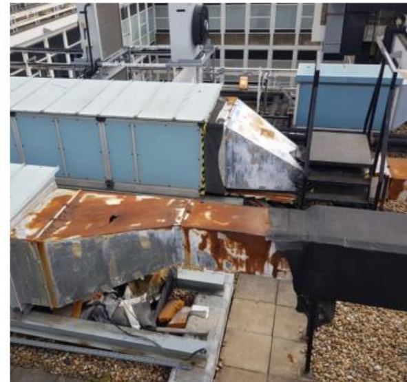
Image 3: Existing Plant on the East Wing Roof
