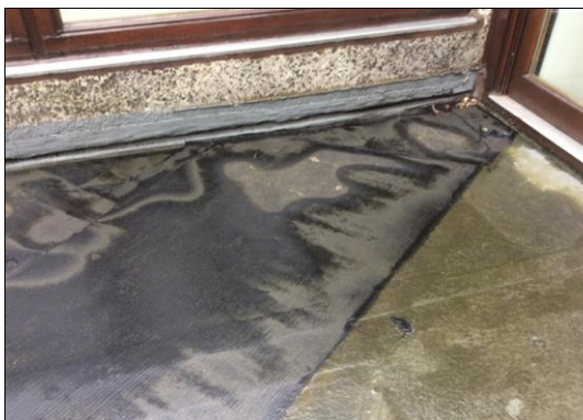
10. Cromwell Tower balcony roof Felt repair has become ruckled and blistered and liquid repairs have taken place to the concrete upstand.
