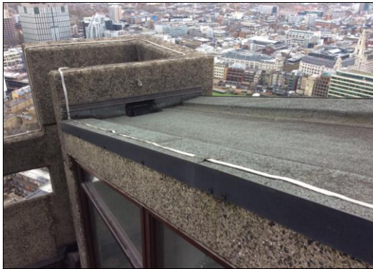
8. Overview of Cromwell and Shakespeare Tower link roofs that are in average condition.
