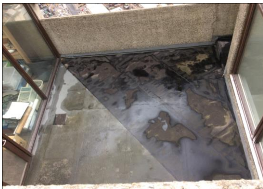
8. Cromwell Tower balcony roof Overview of Cromwell Tower balcony roof; in poor condition and has previous repairs.
