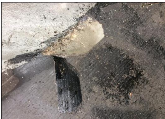
9. Cromwell Tower balcony roof Felt repair has started to fail leaving an aperture for potential water ingress.
