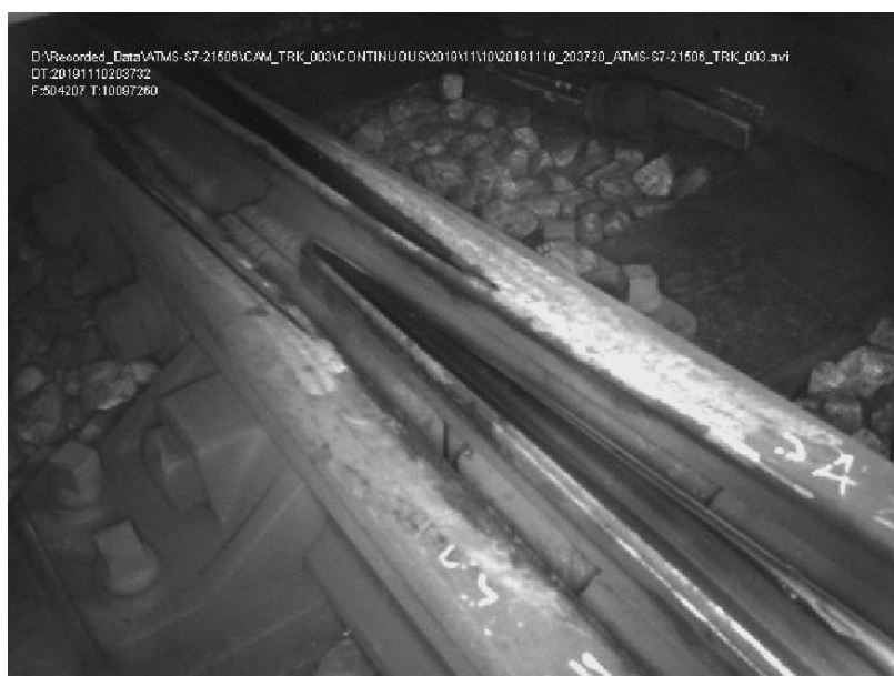
Figure 2 – Rail discontinuity (nose of points 35A) on the right hand rail at LCS M134/MORLO 466m
