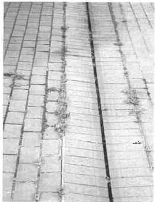
Plants in mortar joints on Cromwell Highwalk
