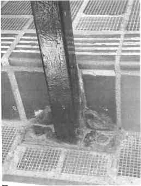
Corroded fixings on steps up to Beech Highwalk from Lauderdale Place
