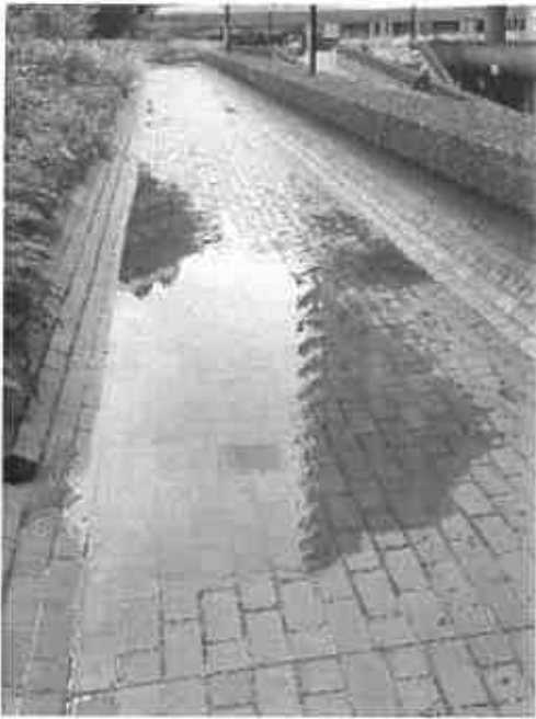
Flooding on the new Beech Gardens Highwalk
