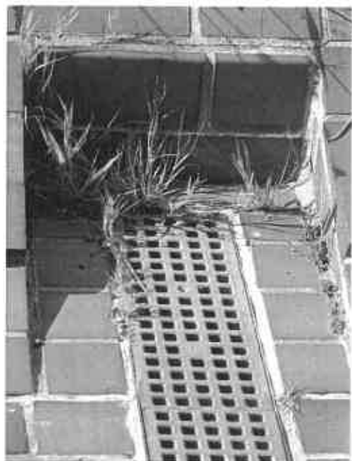
Grass growing out of a drain on Beech Gardens Highwalk
