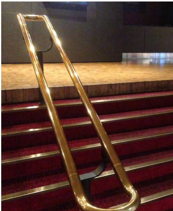
The tubular brass handrail detail and stair nosings, convey a ceremonious opulence
