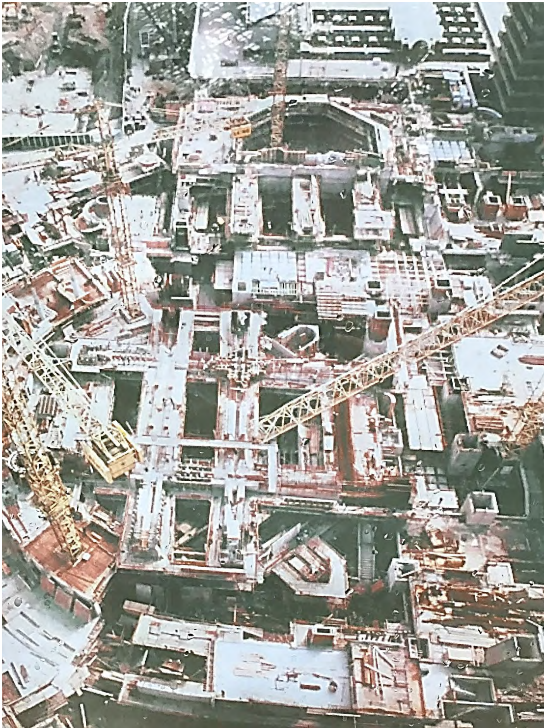
The Barbican Arts Centre under construction, showing Concert Hall (centre), Frobisher Crescent (left) and the Theatre (top)
