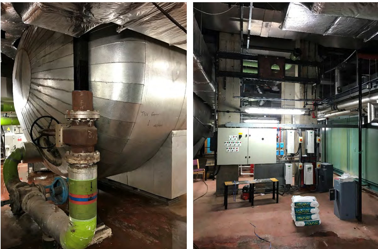
Typical views in the main plant room
