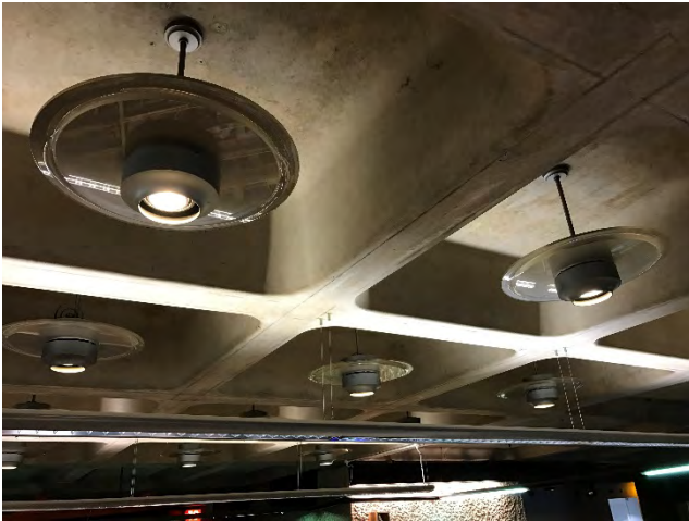
Suspended supplementary lighting tracks
