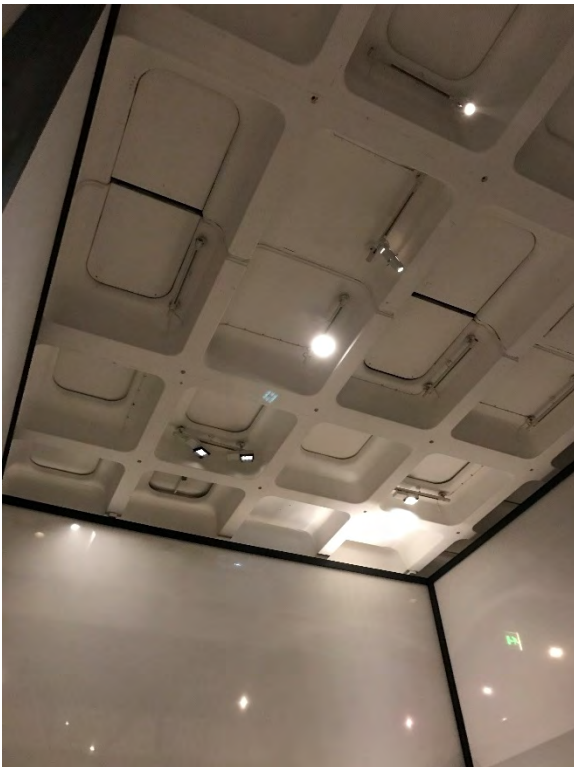
Painted soffit with removable black-out panels
