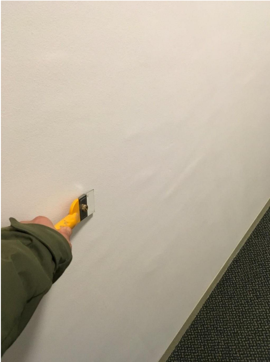
Fig 6, Walls are not smooth and even
