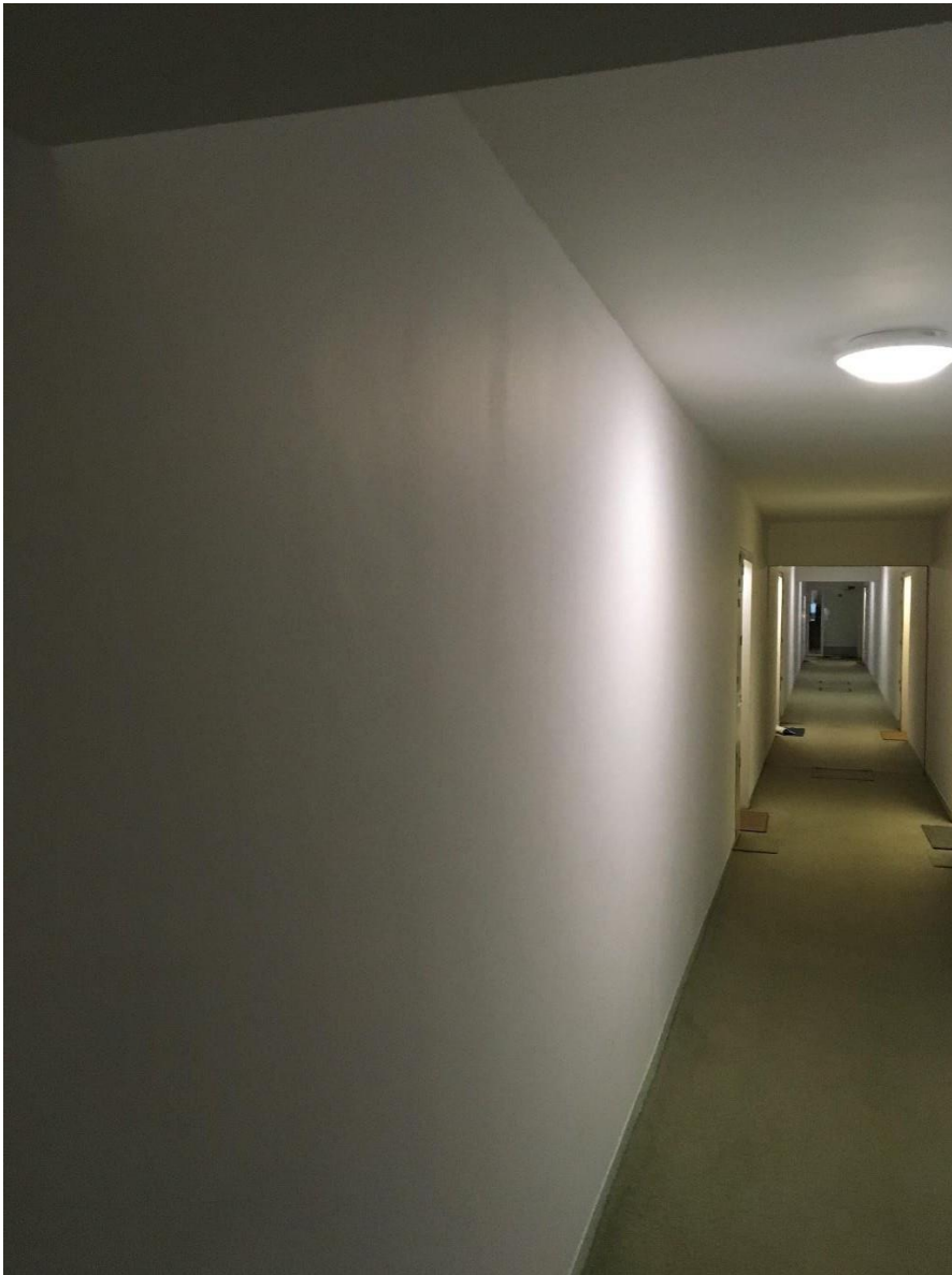
Fig 1, Walls & ceiling affected by critical lighting
