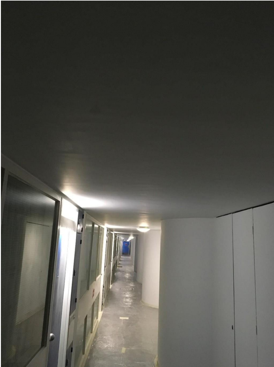
Fig 8, no flashing observed on walls which were curved
