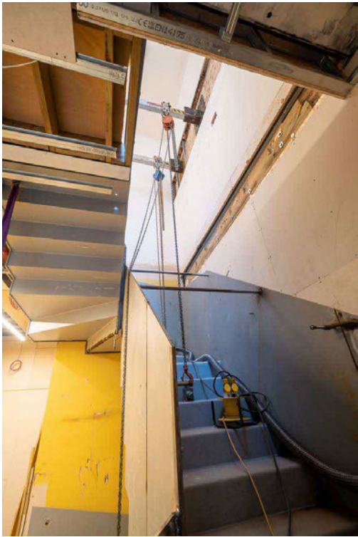
Below: the staircase has been installed to take visitors down to the basement area
