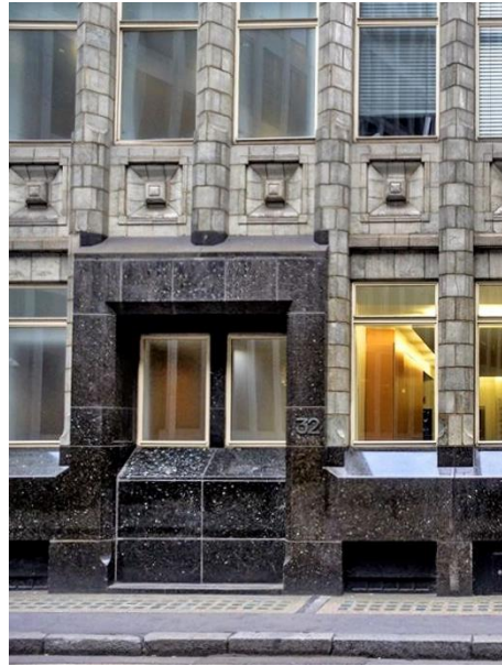
View 2: Entrance to No. 32 currently blocked
