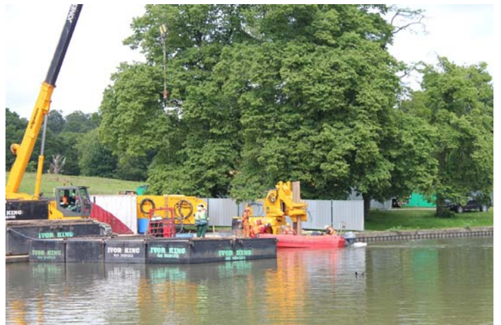
Picture 6 - The piling rig pushing the sheet-metal piles into place using a silent vibration-less technique.
