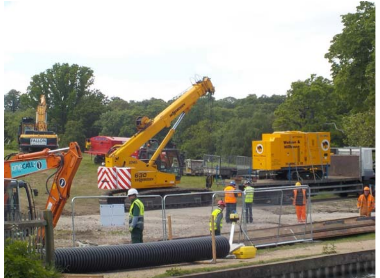
Picture 4 - Forty ton crane being used to move sheet metal piles into place.
