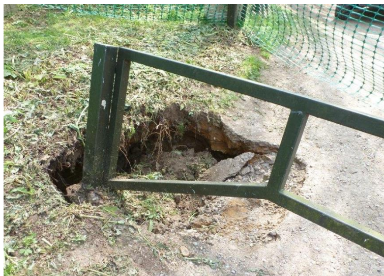
Figure 3: Sink hole at the Vale of Health.
