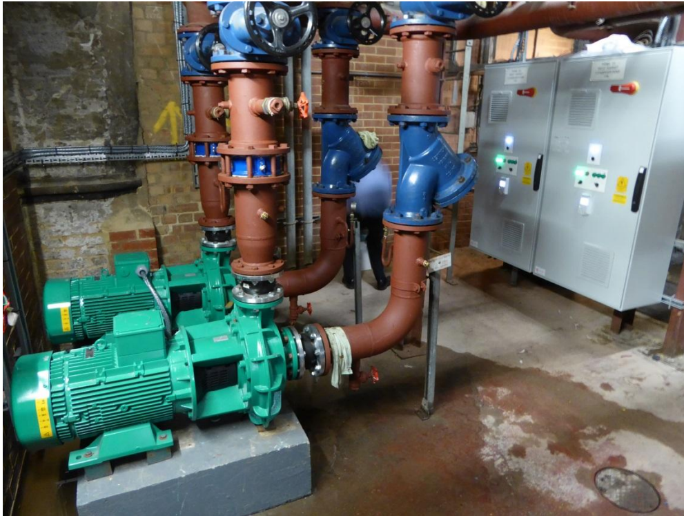
New condenser water pumps and control panels - West Market
